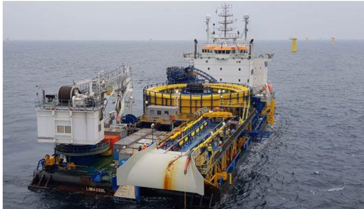
Figure 3.12: Example of inter-array cable installation at the EnBW Hohe See Offshore Wind Farm construction site in the German North Sea.
